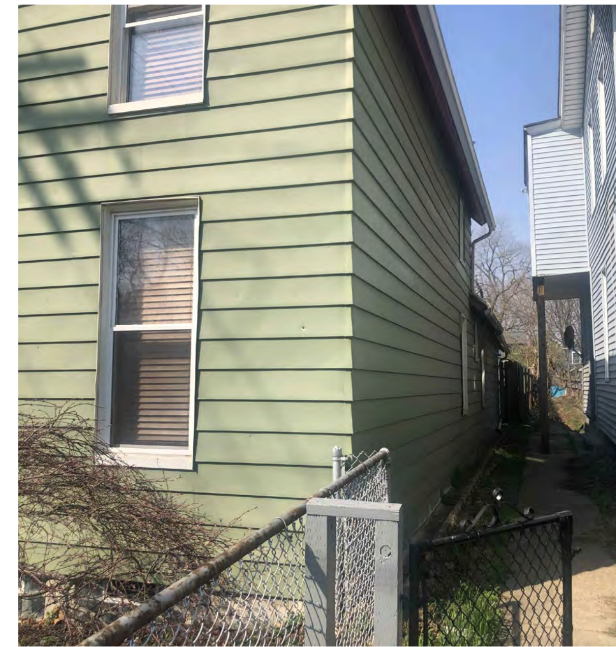
W 44TH STREET - WEST SIDE LESS THAN 3' CLEAR
