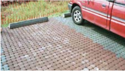
Porous parking and green pavers
