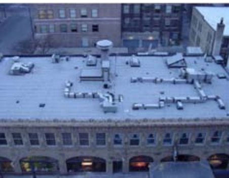
Mechanical equipment setback from the parapet
