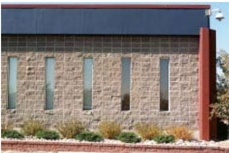
Large expanses of smooth material should be broken up with expansion joints, reveals, or changes in texture or color
