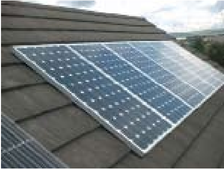
Solar panels on roof for energy generation
