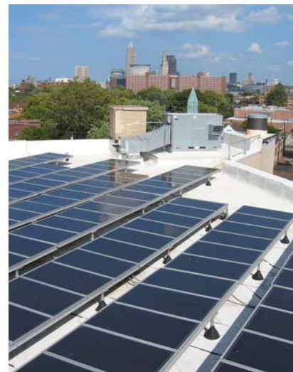
This solar array is one element of the Cleveland Environmental Center's green building attributes. This 1918 bank building is the first commercial, historic green building retrofit project in Ohio and is a national model. [Ohio City neighborhood, photograph by David Beach]
